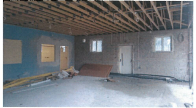
Old hall stripped right back, and the second serving hatch and doorway from new kitchen can be seen towards the corner.
