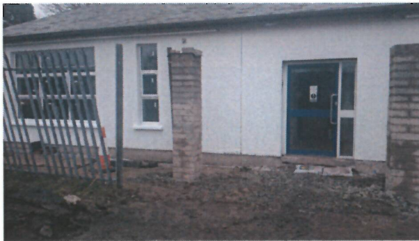
Outside front – new larger windows, pillars in place for new porch at entrance
