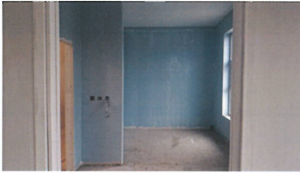
This will be new reception and office viewed through window hatch in entrance hallway. This is located where the old kitchen and one of the small offices were.
