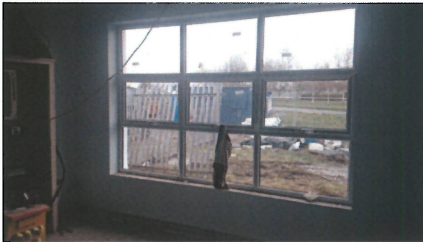
New enlarged room for teenage drop-in. Large windows at front of building make a big difference.
