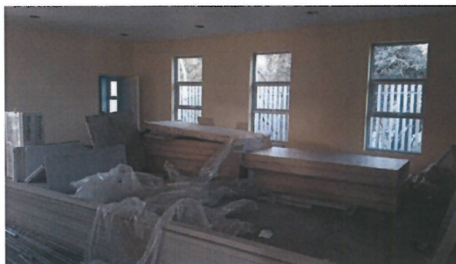
Ignore the insulation and timber-frames! This is the revamped room for younger children, new full length windows, door-way leading to new toilets for kids
