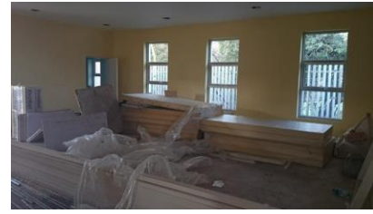
New windows in children's room. Originally, there were only two small windows, each of which was approximately the size of one pane in the new windows.
