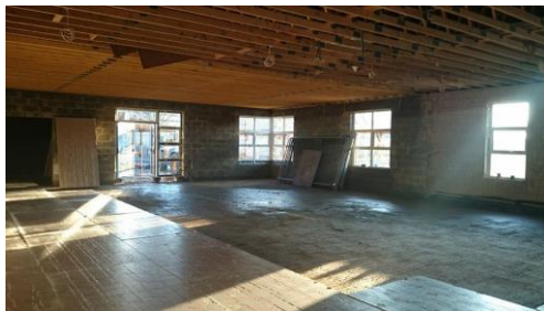
Under-floor insulation being laid in extended hall. New windows and the second new entrance door to hall through gable wall all being installed.
